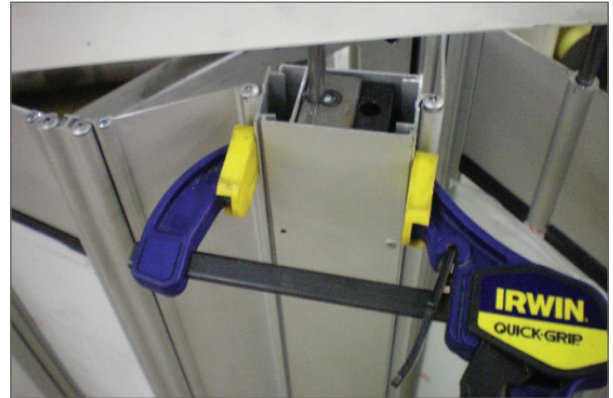
Figure 4: Use of quick clamps to join the post hinge to the post
